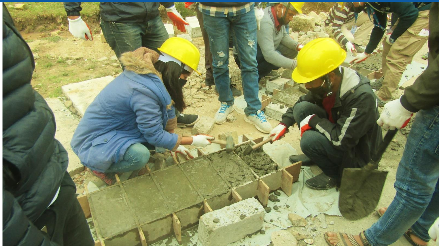
Caption: 4 th Day of training of Mason TOT by NRA/NSET at Bhimeshwore Municipality – 06, Simpani. Participants will be able to conduct refresher training to the working masons after completion of training in coming days.
