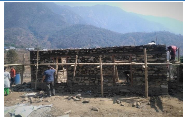
Figure 4: Makwanpur Gadhi Rural Municipality-08, house owner Buddhi Maya Yonjan. Her house is in under construction with stone in mud mortar with RCC band. She has received second tranche.
