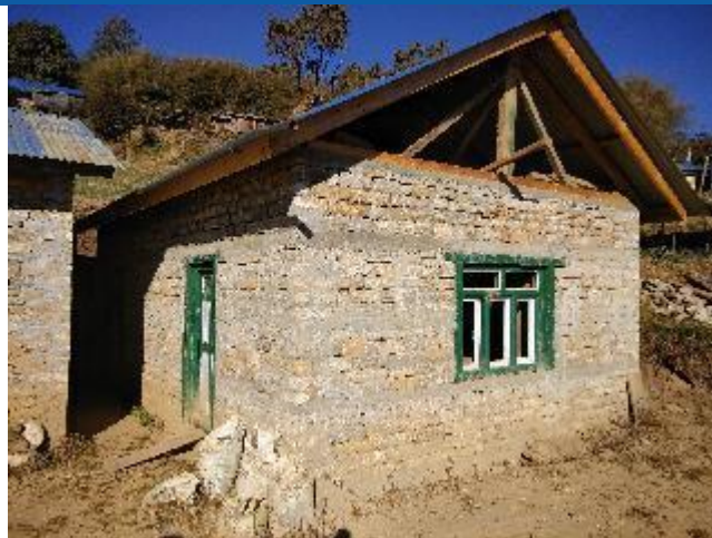
Caption: The house of Furnima Sherpa constructed in Preeti of Umakunda Rural Municipality (4). The house owner has received the second tranche of reconstruction grant. He has taken 2 lakhs as loan from co-operative at 15% interest. The gable wall of light materials is remaining to be constructed
