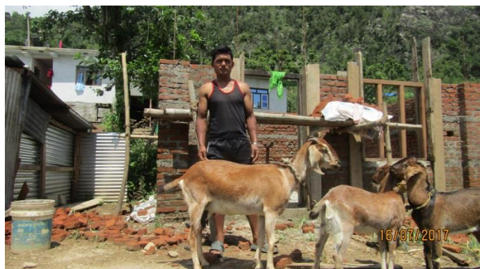
Caption: Kalika Rural Municipality ward no 5, Rasuwa House Owner Name: Hit Badhur Bulun, Construction ongoing, brick masonry, received 2nd tranche.
