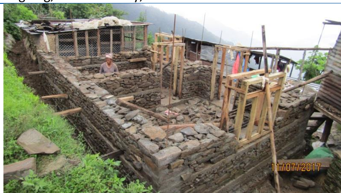
Caption: Kalika Rural Municipality ward no 5, Rasuwa House Owner Name: Jawan singh Bulun, Construction ongoing, stone masonry, received 2nd tranche.
