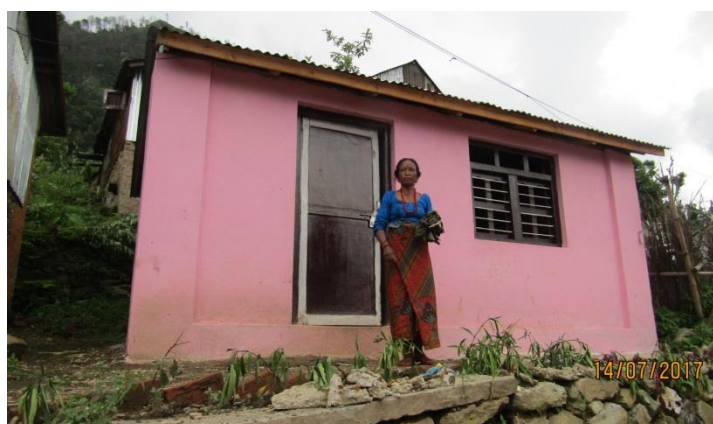
Caption: Kalika Rural Municipality ward no 5, Rasuwa House Owner Name: Kamana singh Bulun, Construction completed, stone masonry, received 3rd tranche.
