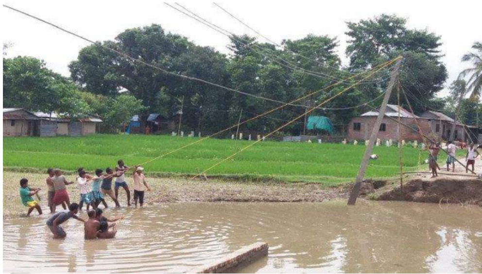
Residents of Taghandubba, Jhapa, try to pull an electricity pole back up after it had been brought down by flooding. Photo credit: Shubhanga Pandey.
