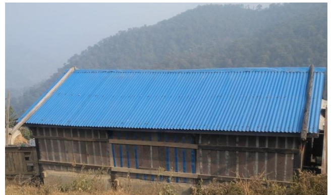
Figure 4: Hybrid structure, ground floor constructed with stone in mud mortar and first floor constructed with timber structure with flexible roof but this building was constructed without supervision of technicians and before 1years. it is non-compliance issues so DSE suggested for correction like as provide vertical post, to provide chicken mesh wire in band with required area. Also we regular flow up this noncompliance issues.
