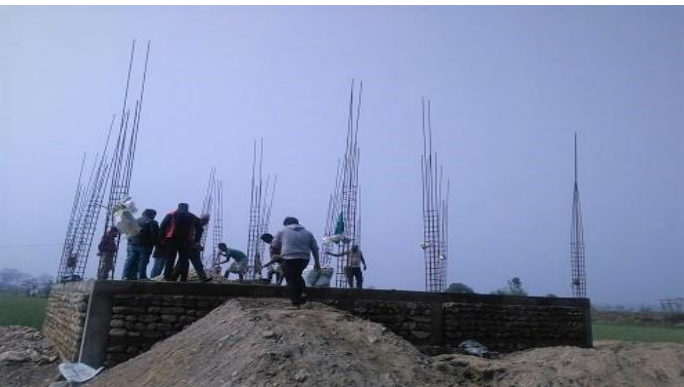
Figure 3: RCC frame structure, house owner is Khadak Man Shrestha. This building is in under construction and recommended for 2 nd tranche by DLPIU field base engineer. location of this building is Manhari Rural Municipality-05.
