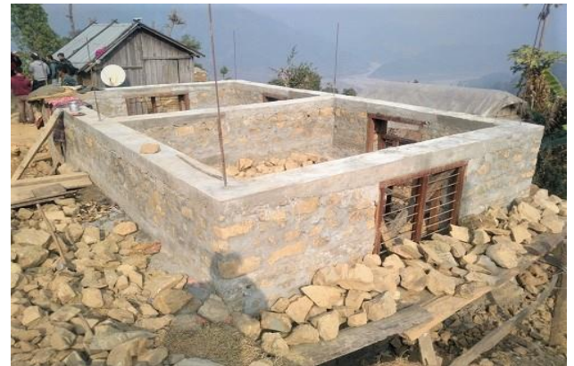
Figure 2: Manhari Rural Municipality, Makwanpur. House owner Shant Bahadur Thokar is made up stone in cement mortar. Under construction building, house owner has received 2 nd tranche and processing for third tranche. Also he has constructed the toilet.
