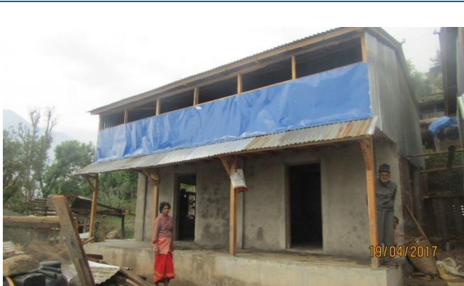
Caption: Kalika Rural Municipality ward no 04, Rasuwa. House owner name: Deep Acharya. Construction completed. Hybrid structure, received all GoN cash support.
