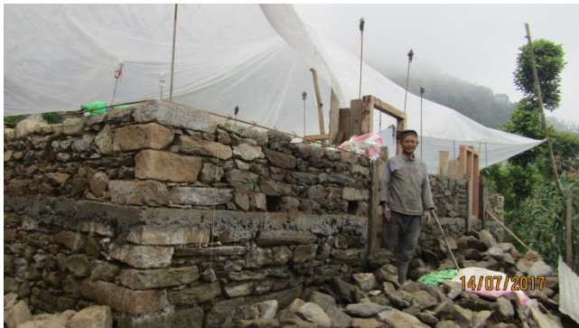
Caption: Kalika Rural Municipality ward no 04, Rasuwa. House Owner: Balkrina Bulun, construction ongoing, received 2nd tranche, stone with cement.
