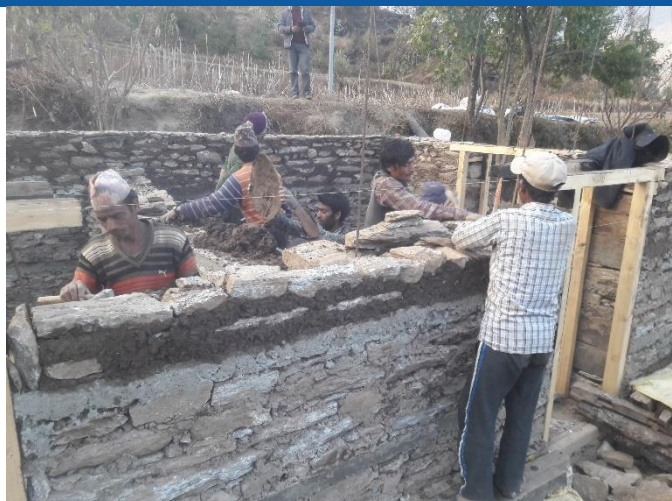
Caption: Masons are working in SMM building in Tamakoshi Rural Municipality, ward-07. House owner had received first tranche and second is in process.
