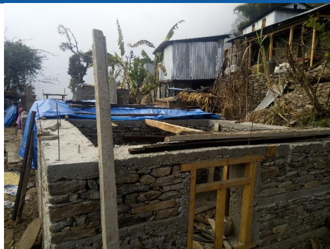
Caption: Dry Stone masonry with RCC band is in construction in Tamakoshi Rural Municipality, ward-06. House owner had received second tranche.
