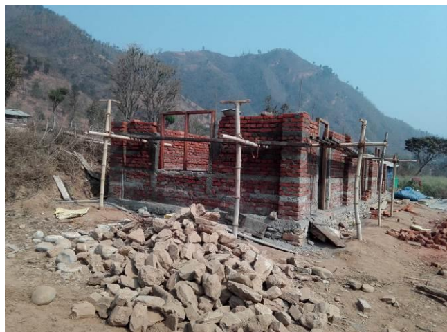
Name :- Bal Kumar Sarki Address: - Kumpur, Siddhalekh Rural Municipality. Type of house:-Brick Masonry in Cement Mortar Approved for 2 nd Tranche
