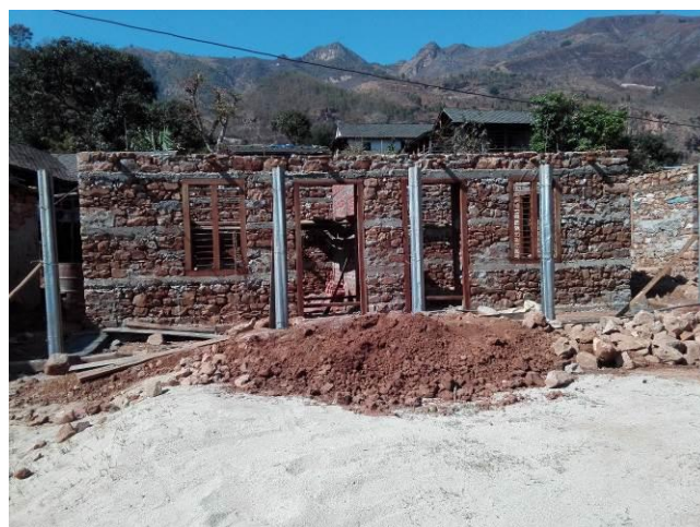
Name:- Durga Badharu Bhandari Address: - Kumpur, Siddhalekh Rural Municipality Type of house:-Stone Masonry in Mud Mortar Get 2 nd Tranche
