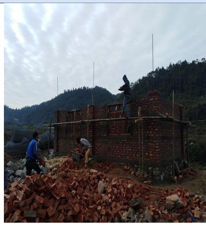
Caption: Brick masonry structure building of Dudhali Municipality ward no – 05 of Sindhuli district. The beneficiary had got 2 nd tranche and construction status of building is in lintel band.
