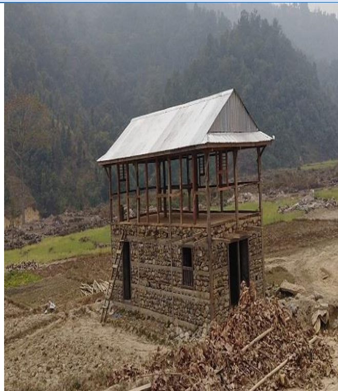
Caption: Hybrid Structure building with lower level massonary structure in Ghanglake Rural Municipality ward no- 03 of Sindhuli district. The building is of two storey and the beneficiary is waiting for government 3 rd tranche.
