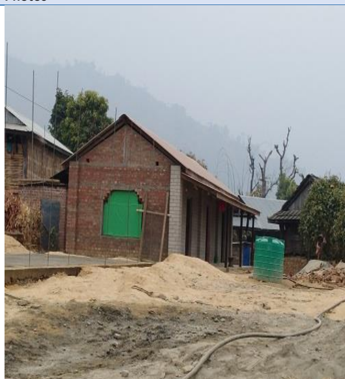
Caption: Brick masonry Structure building of Bastipur ward no-02 of Ghanglake Rural Municipality of Sindhuli district. The house is constructed with gable wall with horizontal and vertical gable bands in appropriate position. Construction of this house is completed and the beneficiary is waiting for 3 rd tranche.
