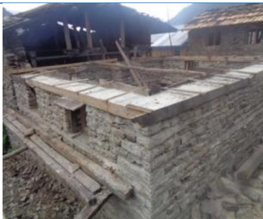
Stone Masonry with cement on Parbatikunda Rural Municipality ward no 4 (Gatlang) Second tranche received. House owner name Mr. KongGong Tamang
