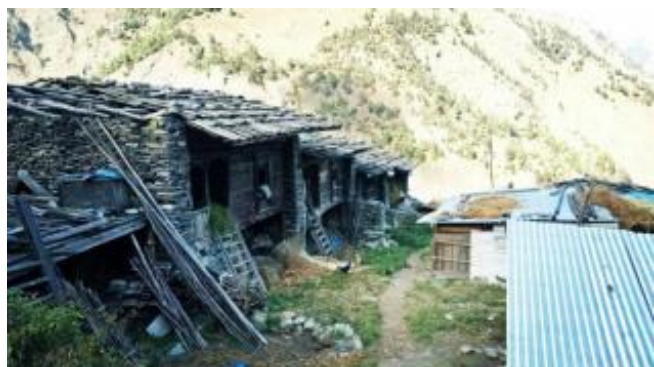
Earthquake affected construction at Parbatikunda Rural Municipality ward no 4.
