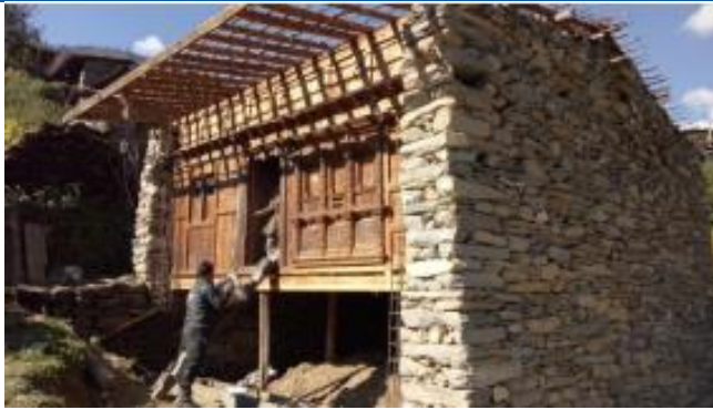
Retrofitting on dry stone masonry. Build change conducting retrofitting on Parbatikunda Rural Municipality ward no 4 (Gatlang)
