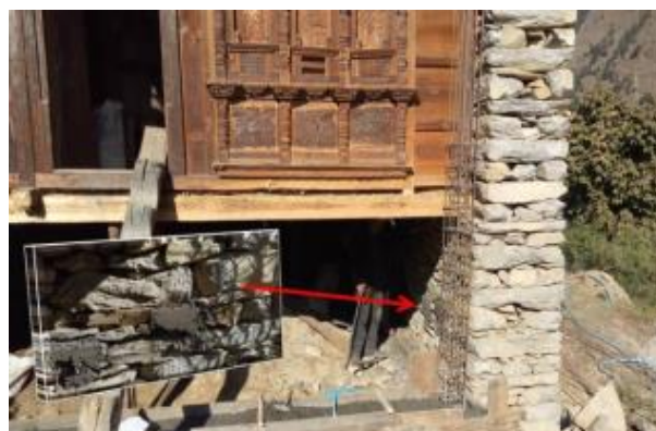
Retrofitting ongoing construction. Build change is conducting retrofitting on drystone masonry at Parbatikunda Rural Municipality ward no 4 (Gatlang).
