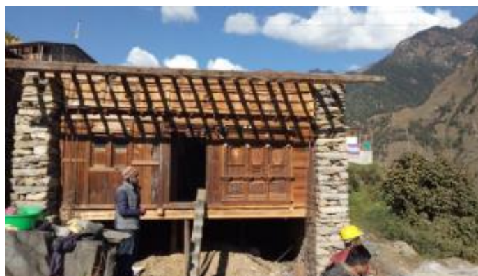
Retrofitting ongoing construction. Build change is conducting retrofitting on drystone masonry at Parbatikunda Rural Municipality ward no 4 (Gatlang).
