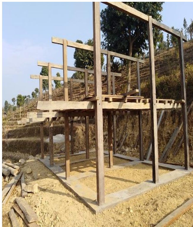
Caption: Wooden frame structure building of Hariharpurgadhi Gaunpalika ward no-01 of Sindhuli district. The house is in DPC level and beneficiary is waiting for 2 nd tranche.
