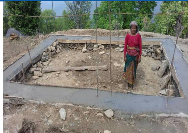
Caption: Siranchowk rural municipality-3, Harmi, Narimaya Nepali's freshly casted plinth band prepared with the support of CARE. CARE is providing top-up support to vulnerable households and making them eligible up-to second tranche level through previously trained mason's refresher training.
