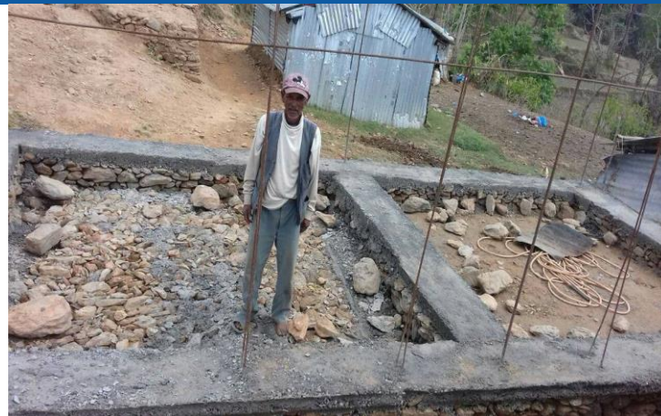
Caption: Siranchowk rural municipality-3, Harmi, Suk bahadur Nepali's freshly casted plinth band prepared with the support of CARE. CARE is providing top-up support to vulnerable households and making them eligible up-to second tranche level through previously trained mason's refresher training.
