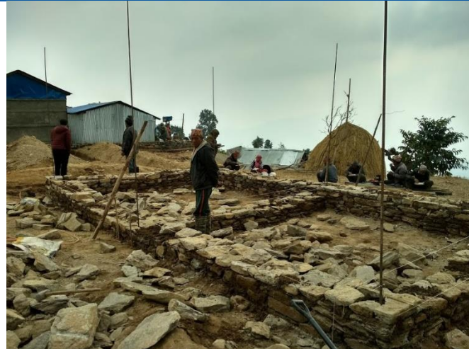
Caption: Mucchok ward no. 5, Ajirkot Gaupalika, Gorkha district, stone masonry foundation of Mr Suk Bahadur Gurung which is ready for plinth beam casting. Mr Gurung is a trained mason, training provided by JICA.
