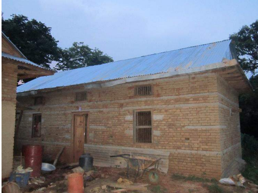
Ojhetar, Panchkhal Municipality: this house has been constructed using adobe bricks and all the required earthquake resistant elements have been included. The house owner has received the municipal permit for the design.
