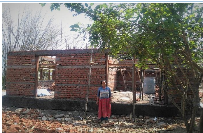
Figure 3: Under construction house, brick in cement mortar with all Horizontal & vertical elements. House owner Kali Bahadur Praja, he received second tranche and process for third tranche. Location of this house is Raksirang Rural Municipality-08.
