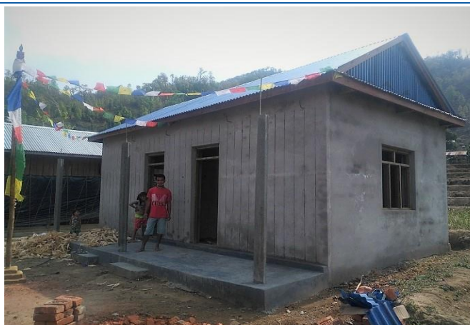
Figure 4: Raksirang Rural Municipality-03, house owner is Lal Bahadur Lama, he received second tranche and verified for third tranche by NRA engineer. All vertical and horizontal elements provided with flexible roof. The total cost of this house is around 5 Lakhs.
