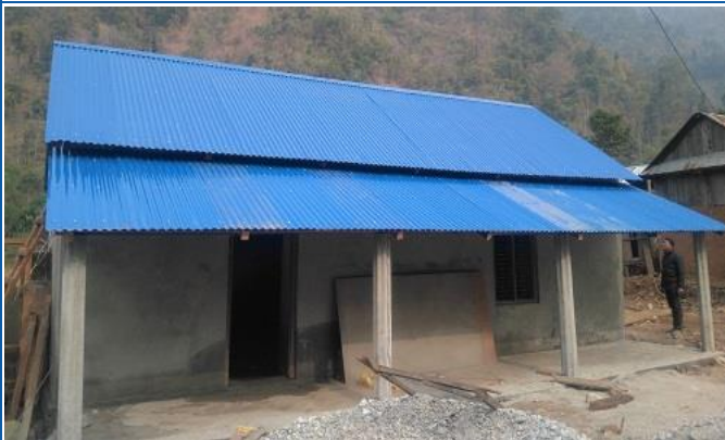
Figure 3: Stone in mud mortar with flexible roof, all vertical post & this house verified for second tranche, third tranche as well. House owner: Kanchi Maya Waiba and location is Sarikhet-01 current Ramsirang RM-03.
