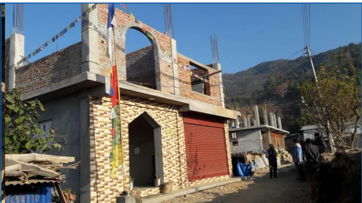
Address: - Semjong, Netrawati Rural Municipality. Type of house:- RCC framed structure building with brick masonry in C/M .
