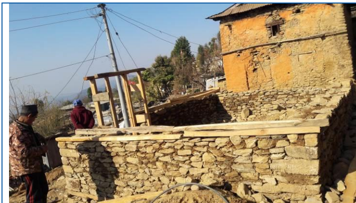
Address: - Gumdi-04, Gangajamuna Rural Municipality. Type of house:- One story load bearing structure, stone masonry in mud mortar with wooden band Received 1 st Tranche, Approved for 2nd Tranche
