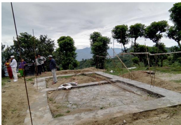
[Ratanchura] [Brick masonry with cement mortar ] [Vertical reinforcement provided but plinth level flushes with ground level])
