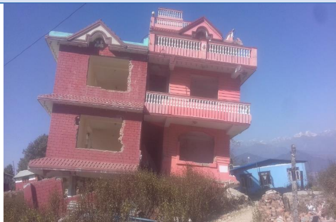
Houses in Haibung are still undismantled as such technology are not available there. This house lies in Chisopani, Haibung, which is a famous trekking route, it is at a risk of collapsing anytime, and the route lies underneath it, which is a threat to trekkers.
