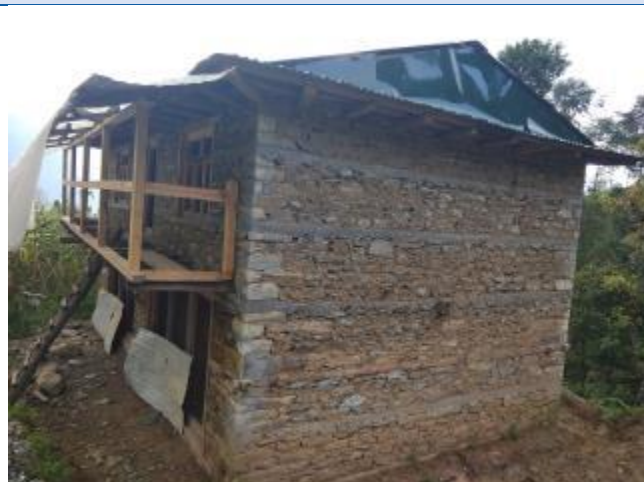
Caption: House of Uday Tamang of Shreechaur VDC. The house owner has received second tranche of reconstruction grant. The house has been completed upto 2 floors with RC band.
