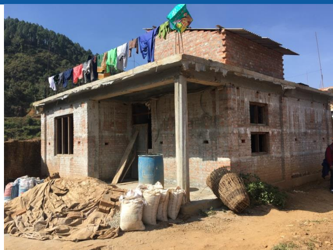
Chapagaun Ward no. 10, 3 rooms single storey Load bearing structure with RC roofing. The reconstruction of the house in almost complete.
