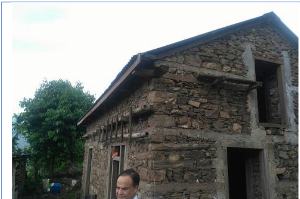
Stone in mud mortar with flexible roof with RCC band 1st and 2nd tranche received and processing on third tranche ,owner Aaite sing Tamang N-27 27 56 E 85 2 43
