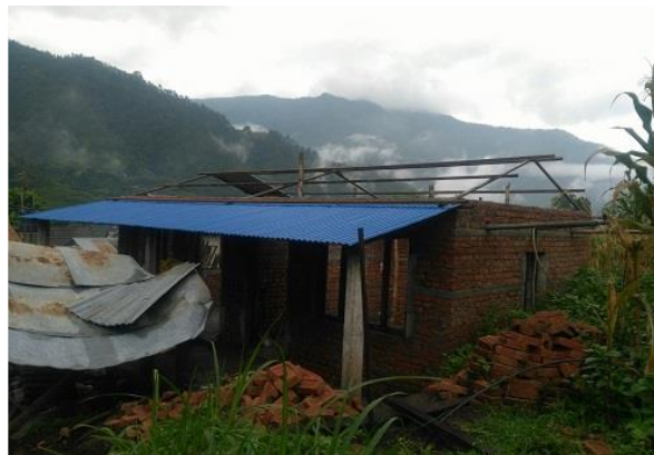
Below plinth, stone in mud and above plinth brick in cement mortar with flexible roof at Bhimfedi Gaupalika 3 (Nibuwatar 08) ,owner Praseep Tamang N-27 1 24 E 85 5 07
