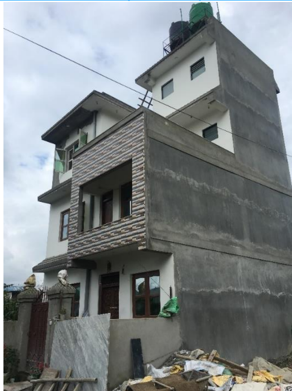
Ward No.9, Chandragiri Municipality, Kathmandu: three storey, RC frame structure. Lumanti are providing support to the home owner who had faced issues due to conflict regarding ownership of the land but has now been able to proceed with the housing reconstruction grant process.
