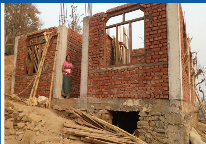
Caption: Gorkha Municipality ward no 6, under construction R.C.C frame structure of Bhakta Bahadur Ghale.
