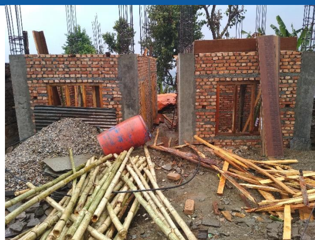
Caption: Simjung, Ajirkot Rural Municipality ward no 4, under construction R.C.C frame house of Ganga Bahadur Gurung. This house has been recommended for second tranche.
