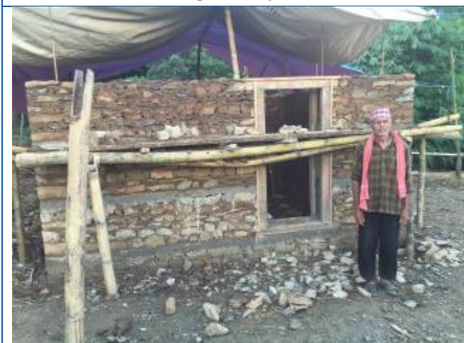
Caption: The house of Shiva Prasad Gautam being constructed in Saipu, Likhu Tamakoshi Rural Municipality-2. The owner has received second tranche of reconstruction grant.
