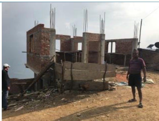
Caption: The house of Raju Dilauri being constructed in Saipu, Likhu Tamakoshi Rural Municipality-2. The owner has received first tranche of reconstruction grant.
