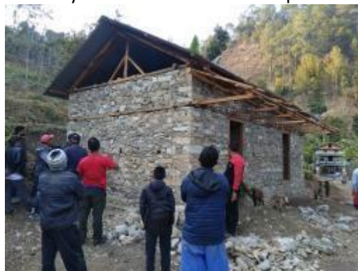
Figure 2. The demo house constructed in Saipu on technical assistance from KAM For SUD Nepal
