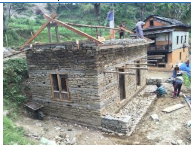
Caption: The house of Hom Bahadur Tamang being constructed in Saipu, Likhu Tamakoshi Rural Municipality-2. The owner has received second tranche of reconstruction grant.
