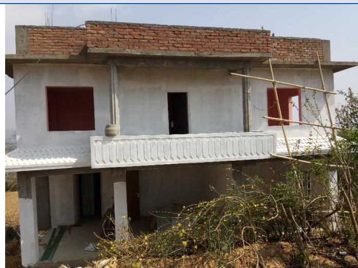
Devasthan, Ward No. 8, Chaimale, Dakshinkali Municipality, RCC frame structure building. The house owner has forwarded the file for 2 nd tranche claim.
