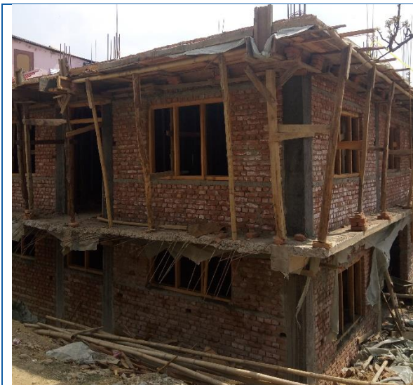
Kaji Gaun, Ward no. 8, Dakshinkali Municipality, RCC frame structure house. The house owner has claimed 2 nd tranche at municipality with all necessary documents, however the monitoring revealed that the area has been exceeded during the construction.
