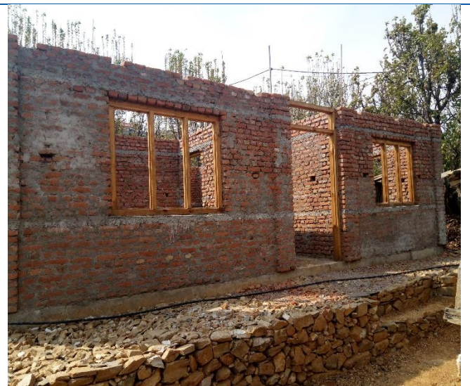
Kaji Gaun, Ward no. 8, Dakshinkali Municipality, wall system house with planning of cement casting on roof. The house owner was recommended to prepare documents to claim 2 nd tranche.
