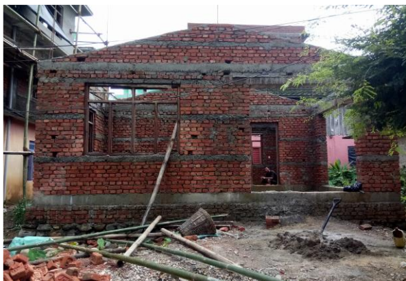
[Brick masonry with cement mortar bands provided with flexible roof, Kamalamai-6 Sindhuli]
