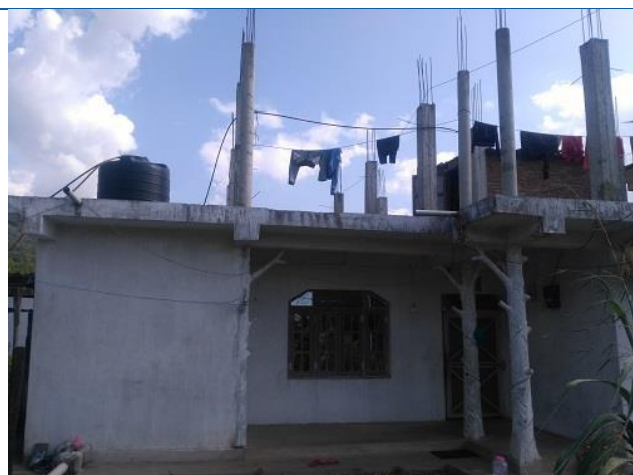
Figure 3: noncompliance building and file sent for structural analysis and located at Manhari Gaupalika.
