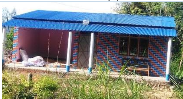
Caption: Block masonry construction and after analysis of SAP by DSE, this house is recommended for second and third tranche and also proposed for shutter in left side of building. House owner: Padam Paudel. The location of building is Manari 06 (Current Manhari Gaupalika 03).
