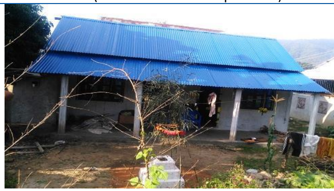
Caption: Block masonry construction and after analysis of SAP by DSE, this house is recommended for second and third tranche. House owner: Shyam Pathak. The location of building is Manari 06 (Current Manhari Gaupalika 03).
