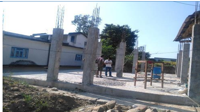
Caption: RCC frame structure with brick masonry at Manhari 07 current Manhari Gaupalika 09. Verified for second tranche. Owner: Khem Raj Ojha.
