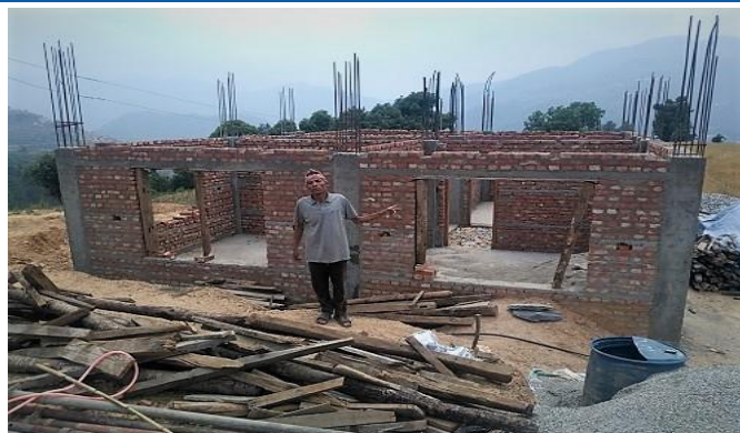
Figure 4: RCC frame structure with meet all mandatory requirement Thumb rule. His house verified for second tranche and the location of building is Indrasarowar-01, house owner name is Ram Sharan Bist.
