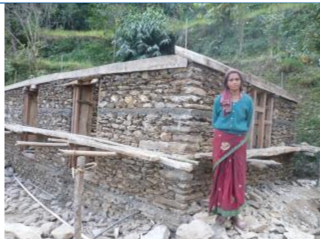
The house of Gunj Bahadur Rawat of Saipu VDC of Likhu Tamakoshi Rural Municipality under construction. The house owner has received second tranche of reconstruction grant. The house is made with stone with mud mortar providing RC bands. The house has been completed upto lintel band. The house has been constructed under the technical support from KAM For SUD Nepal.
