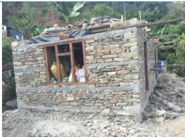
The house of Fulman Tamang of Saipu VDC of Likhu Tamakoshi Rural Municipality under construction. The house owner has received second tranche of reconstruction grant. The house is made with stone with mud mortar providing RC bands. The house has been completed upto lintel band. The house has been constructed under the technical support from KAM For SUD Nepal.
