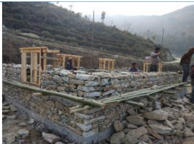
Caption: The house of Durga Bahadur Shrestha, resident of ward number 7, Khadadevi, Khadadevi Rural Municipality being constructed using stone in mud mortar. The RC Bands have been provided to the house. The owner has received the second tranche on magh and is expected to be completed by end of falgun.
