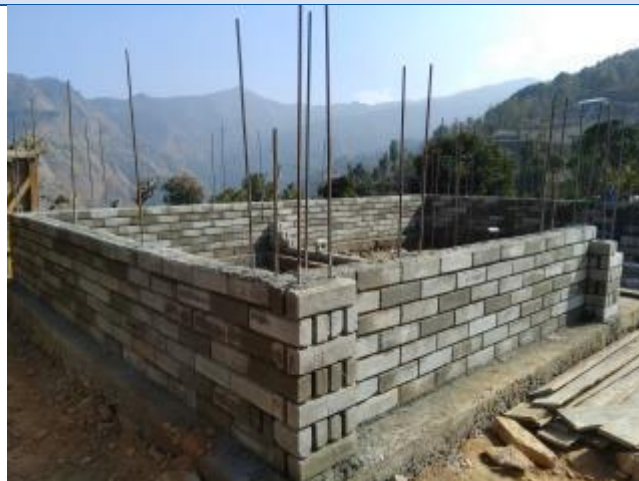
Caption: The two room structure of Garud Singh Tamang, resident of Hiledevi, Sunapati Rural Municipality-3 being constructed by using CSEB interlocking bricks. The blocks are produced by vendor in Mulot and have been constructing the earthquake resilient house at 6.5 Lakhs with free transportation within 10 km area. The house owner has received first tranche. Since he had constructed the plinth level after the Poush end deadline, he has not been verified for second tranche and not been able to receive the second tranche
