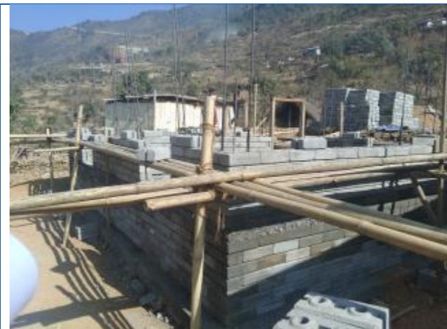
Caption: The two room structure of tranche Keshar Bahadur Shrestha, resident of Bhirpani, Khadadevi Rural Municipality-3 being constructed by using CSEB interlocking bricks. The blocks are produced by vendor in Mulot and have been constructing the earthquake resilient house at 6.5 Lakhs. The house has been recommended for second tranche on Poush 2074 and has not received the tranche yet.
