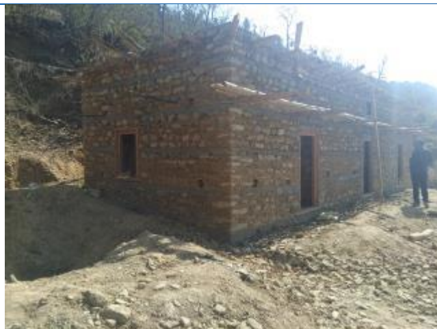
Caption: The three room house of Tek Bahadur Thapa, resident of ward number 3, Bhirpani, of Khadadevi Rural Municipality. The house is being constructed using stone in cement mortar. The RC bands have been provided to the house. He has received second tranche of reconstruction grant on 2 nd Poush 2074. The house is expected to be completed in 8 lakhs.
