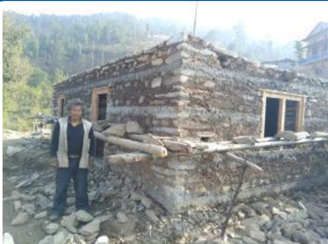
Caption: The two room structure of Brish Bahadur Tamang, resident of former Khadadevi VDC being constructed using stone in mud mortar. The RC Bands have been provided to the house as seismic parameters. He has received second tranche on first week of Asar 2074.
