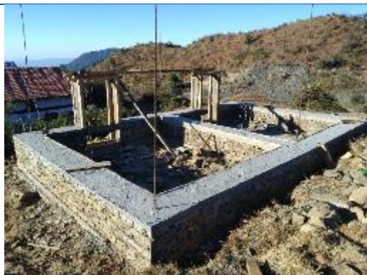
Caption: The house of Krishna Prasad Acharya being constructed on Priti. He have received first tranche of reconstruction grant and has been forwarded for second tranche.
