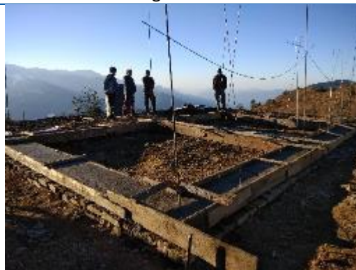
Caption: The house of Dhan Raj Lamichhane being constructed on Priti. He have received first tranche of reconstruction grant and has been waiting for the process for the second tranche by technical personnel.
