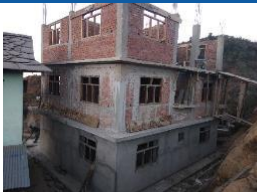
Caption: The house of Man Bahadur Khatri being constructed on Priti of Umakunda Rural Municipality.
