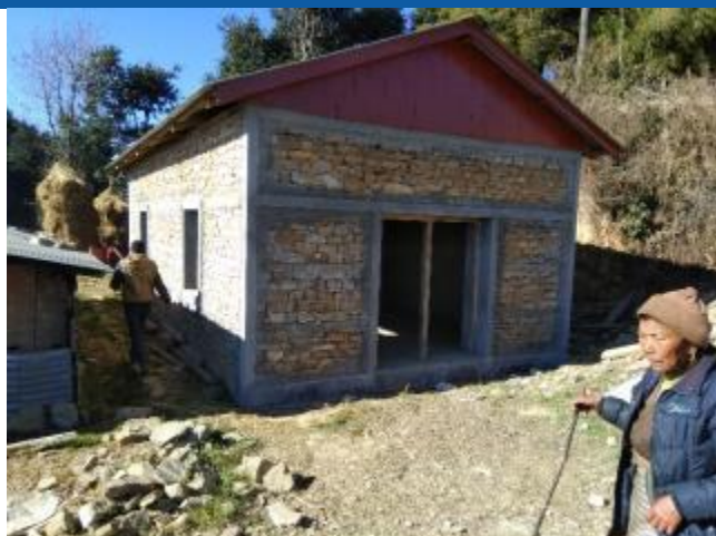
Caption: The house of Pemba Sherpa constructed in Umakunda Rural Municipality-4. The owner has received second tranche of reconstruction grant.
