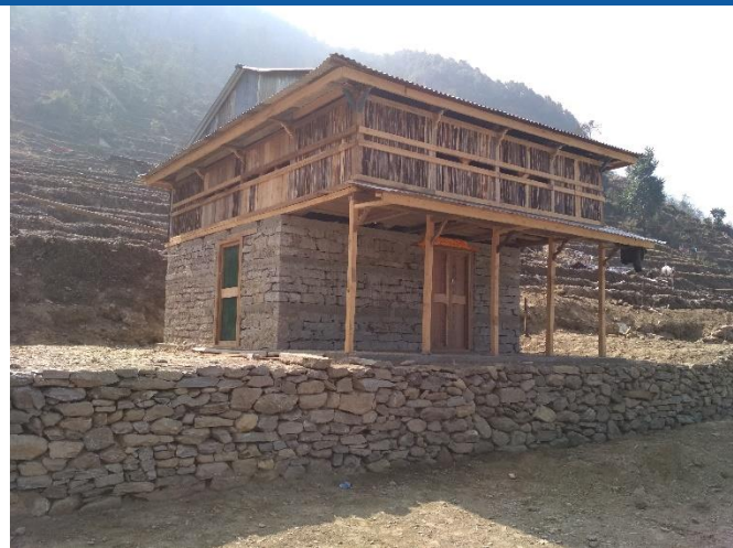
Caption: Polchet, Manbu, Aarughat gaunpalika ward no 1, stone masonry mud mortar house with r.c.c band house with light wooden plank super structure house of Mr. Ram Narayan Gurung. He is yet to receive second tranche although his file has been send to the district
