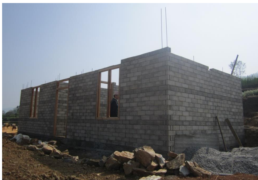
A two roomed Masonry Structure using Interlocking blocks at Kushadevi, Panauti Municipality. The house owner Dambar Bahadur Tamang is a Retrofit beneficiary but as the house was not livable, has applied for switching into Reconstruction beneficiary.
