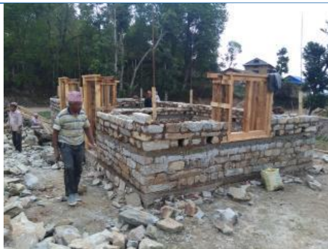
Caption: The house of Nar bahadur Magar of Dimipokhari of Sunapati Rural municipality-2. The house has been constructed using stone in mud mortar. RC band has been provided to the house. The house consists of two rooms. The owner has received second tranche of reconstruction grant.
