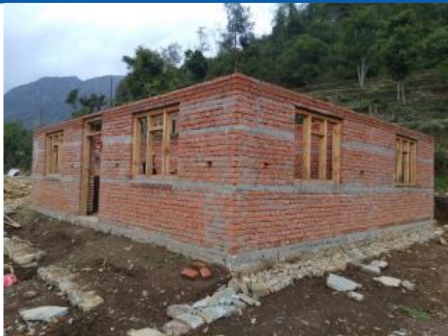
Caption: The house of Manmaya Magar of Dimipokhari, Sunapati Rural Municipality-2 being constructed. The house has been constructed using brick in cement mortar. The house consists of four rooms. The house has been provided with passage of 4'. The doors have been installed within 2' from the corners. The door and windows have not been provided at the same level. The owner has not received any tranches of reconstruction grant.
