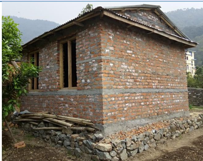
Sisneri, Ward No. 9, Lamatar, Mahalaxmi Municipality, BMC structure with gable band and CGI roof. The house owner has approved building drawing and the house meets the minimum requirements of 1 room house. The owner has received 2 nd tranche.
