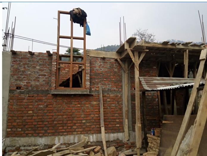
Sisneri, Ward No. 9, Lamatar, Mahalaxmi Municipality, wall system house with cement casting on top. The owner has applied for 2 nd tranche.
