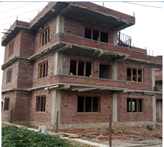
Sisneri, Ward No. 9, Lamatar, Mahalaxmi Municipality, RCC structure house with use of band and cladding in door and windows. The owner has applied for 2 nd tranche.
