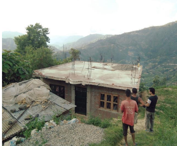
Thakre VDC, Dhading, One storey RCC Building, The beneficiary has received only first tranche.
