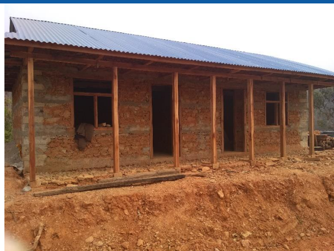
Caption: Jyamiswara - 6, Ghairung of Sahid Lakhani Rural Municipality, completed stone masonry mud mortar house with RCC band and wood beam frame. House owner is Mr. Kumar Rana. He has received second tranche and has been recommended for third tranche.
