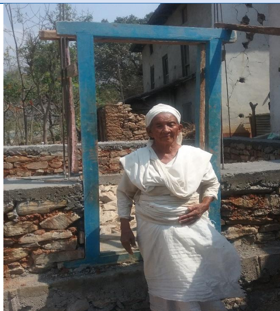
Caption: A Widow woman is in front of her under construction house.
